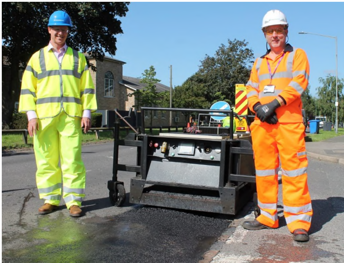
Cllr Geoff Hill (left) sees firsthand the effectiveness of infrared repairs on our highways
